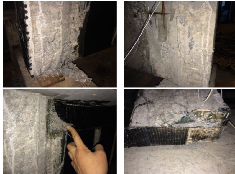
Fig. (9). The failure mode of Team YJG-1.
